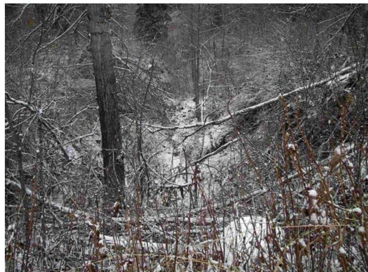
Photo 4 – Eroded trib. Channel below 1000 mm culvert
