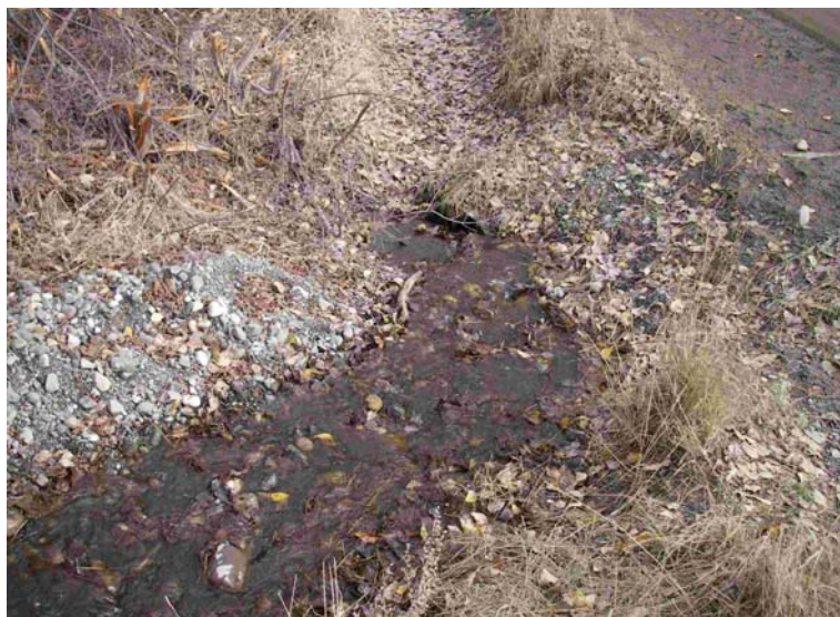
Photo 43 – Barker Creek partially blocked culvert at 100 Rd.
